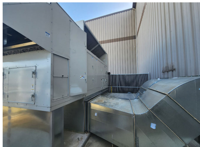
Restrictive duct geometry at the project site necessitated an innovative airflow measurement solution.
